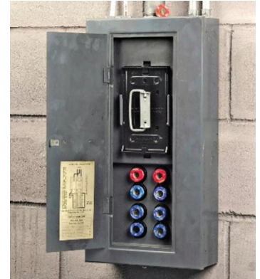
Fuse box style panel
