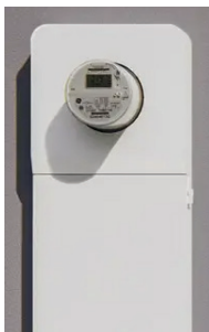
Smart electrical distribution panel
