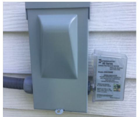
Figure 3: External surge protector
