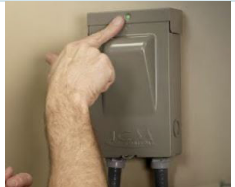
Figure 2: Integrated electrical disconnect with surge protector
